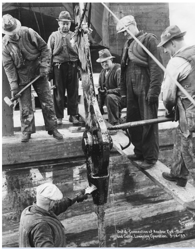
Workers connect an anchor eye-bar and cable, Sept. 14, 1939. Photo: Washington State Archives.
